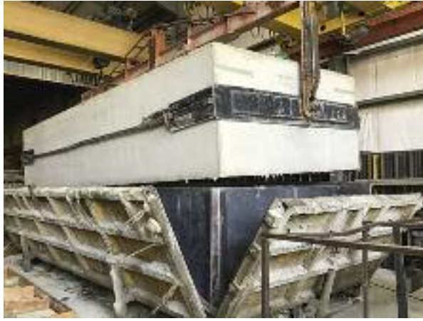
A 40-ton, 50,000 litre concrete septic tank is lifted away from its form at Newmarket Pre-Cast after setting overnight.
