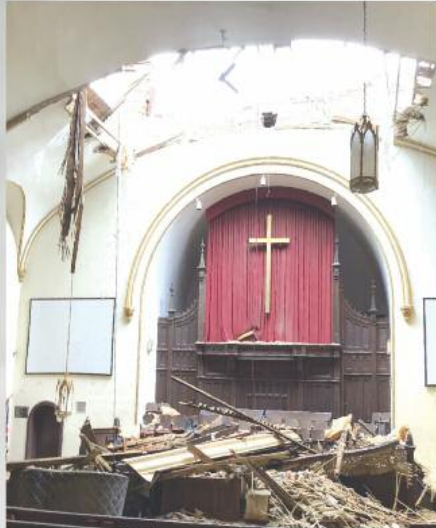
Damage to Trinity United Church was too extreme to see the church restored.
